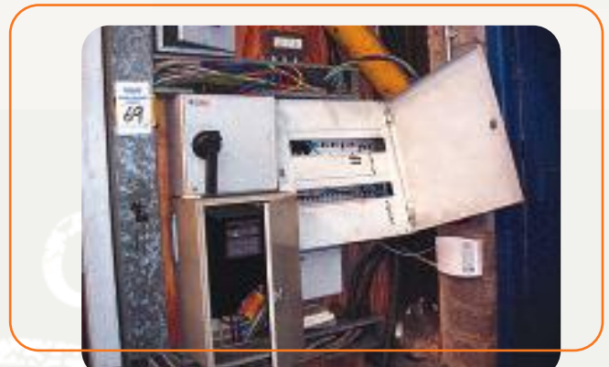
Figure 4 Installations like these can lead to inadvertent contact and electrocution.
