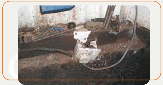
Figure 2 Dangerous electrical outlet giving rise to risk of electrocution
