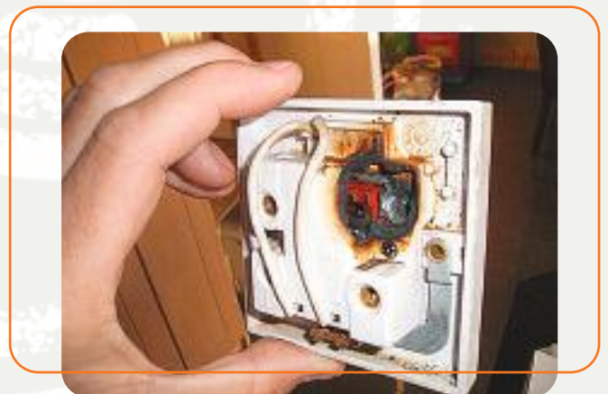
Figure 3 Potential ignition source from electrical equipment
