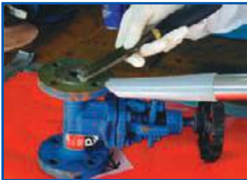
Use of shadow vacuuming to capture dust released in cleaning asbestos from a valve
