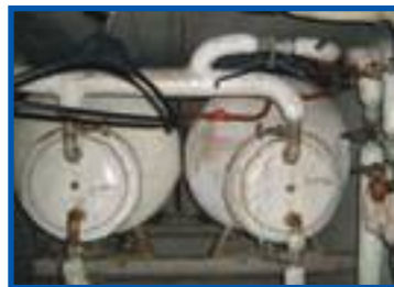
Thermal insulation to calorifier
