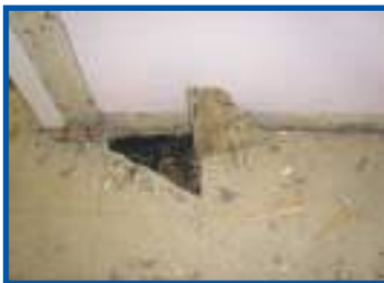
Chrysotile-based floor tiles and chrysotile containing adhesive
