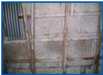
Asbestos spray coating to metal corrugated roof
