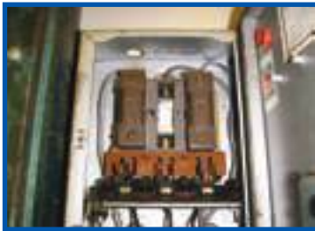
Chrysotile flash guards in old fuse box
