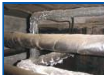
Composite asbestos lagging to pipework in very poor condition
