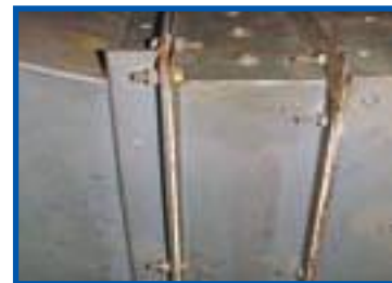
Chrysotile rope seals to flanges of ductwork
