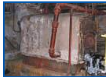
Thermal insulation to boiler
