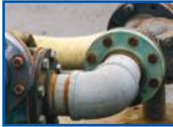
Compressed asbestos gaskets to pipework flanges
