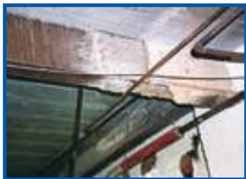
Asbestos spray coating to Rolled steel joist
