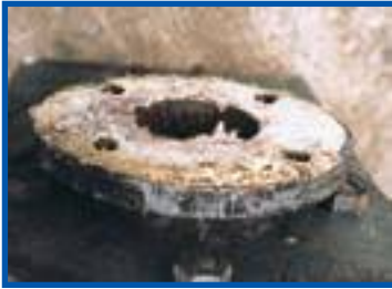
Exposed chrysotile-based compressed asbestos gasket to flange
