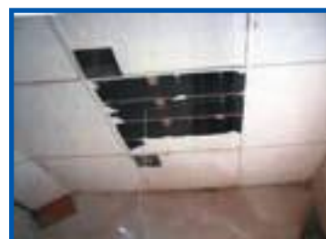
Damaged AIB ceiling panels
