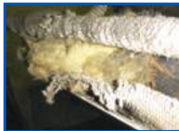
Chrysotile rope lagging to pipework
