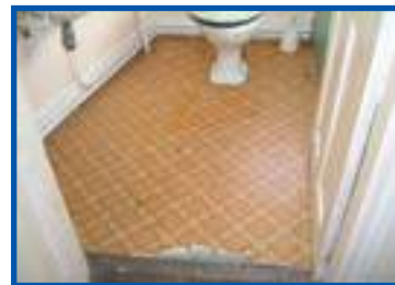
Chrysotile backing to linoleum floor covering
