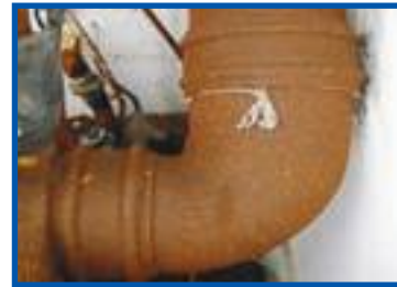
Chrysotile rope to metal boiler flue
