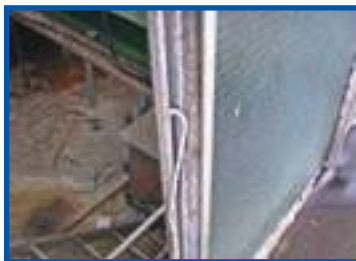
Chrysotile rope seals in glazing units
