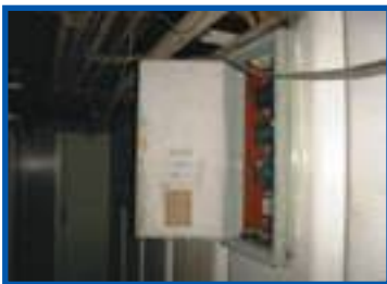
AIB to fuse panel door
