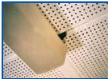
Perforated AIB ceiling panels with minor damage at light fitting
