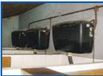
Asbestos-containing shires lynx toilet cisterns
