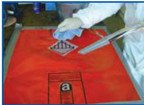
Cleaning up the work area carefully with H-Type vacuum cleaner and wet waste rags
